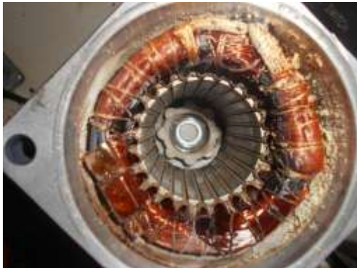
PORT ACTUATOR MOTOR (MOTOR BURNT & SHORTED)
